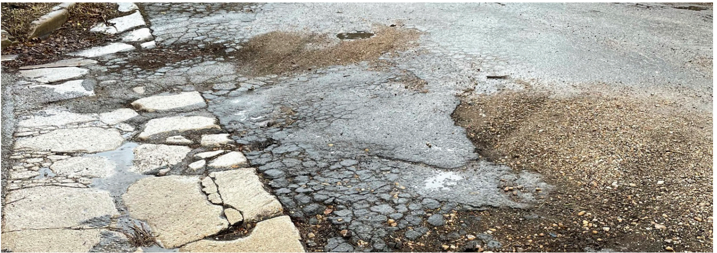
Poor Pavement Conditions, Taylor Texas
