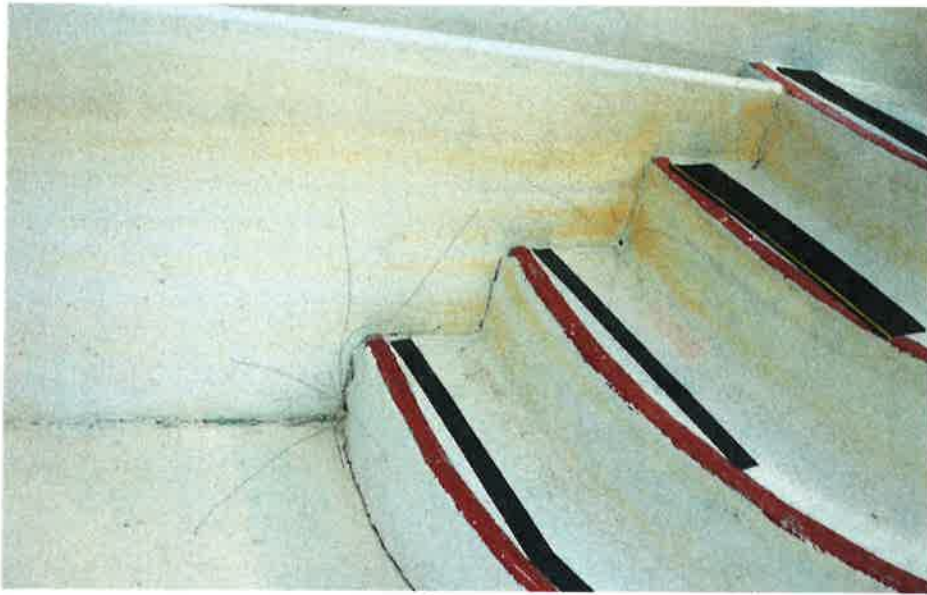
Arrows point to locations of pool leaks near entry steps
