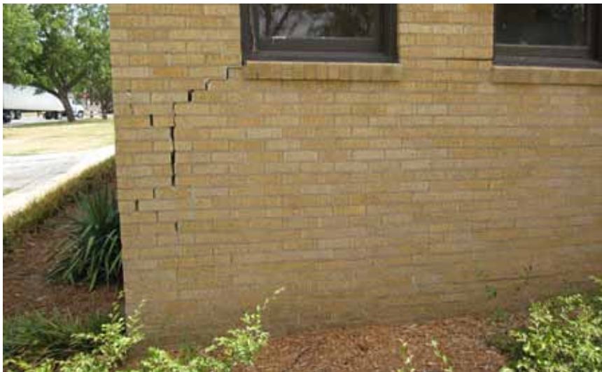
Cracking at northwest corner
