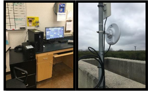
New WWTP SCADA System
