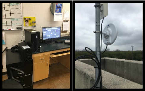
New WWTP SCADA System
