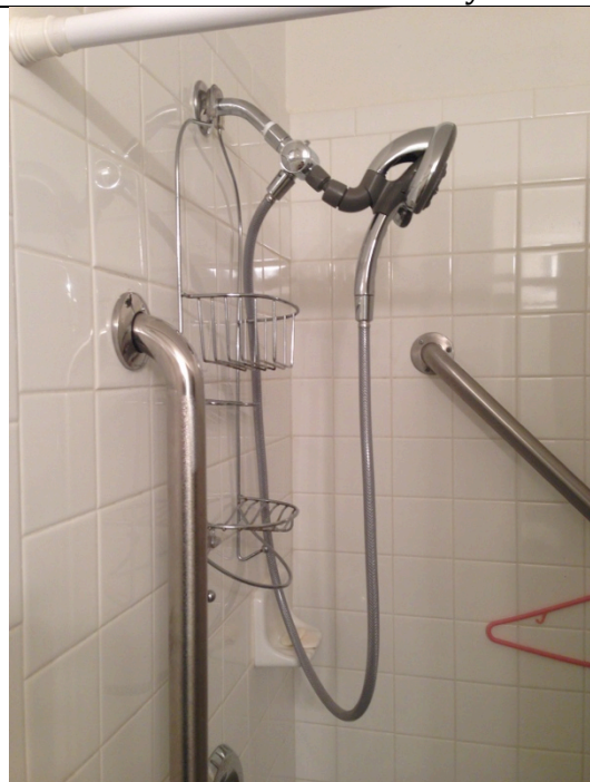
New shower wand. Note tightened grab bars.
