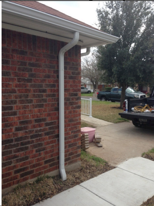
Rain gutters with dual downspouts at northwest quadrant (location of drainage issue).
