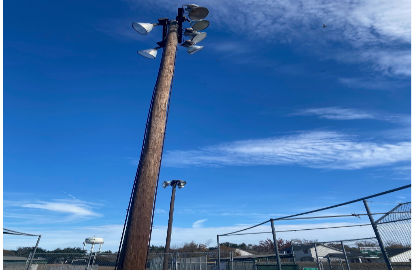
Existing lighting at Bull Branch Fields
