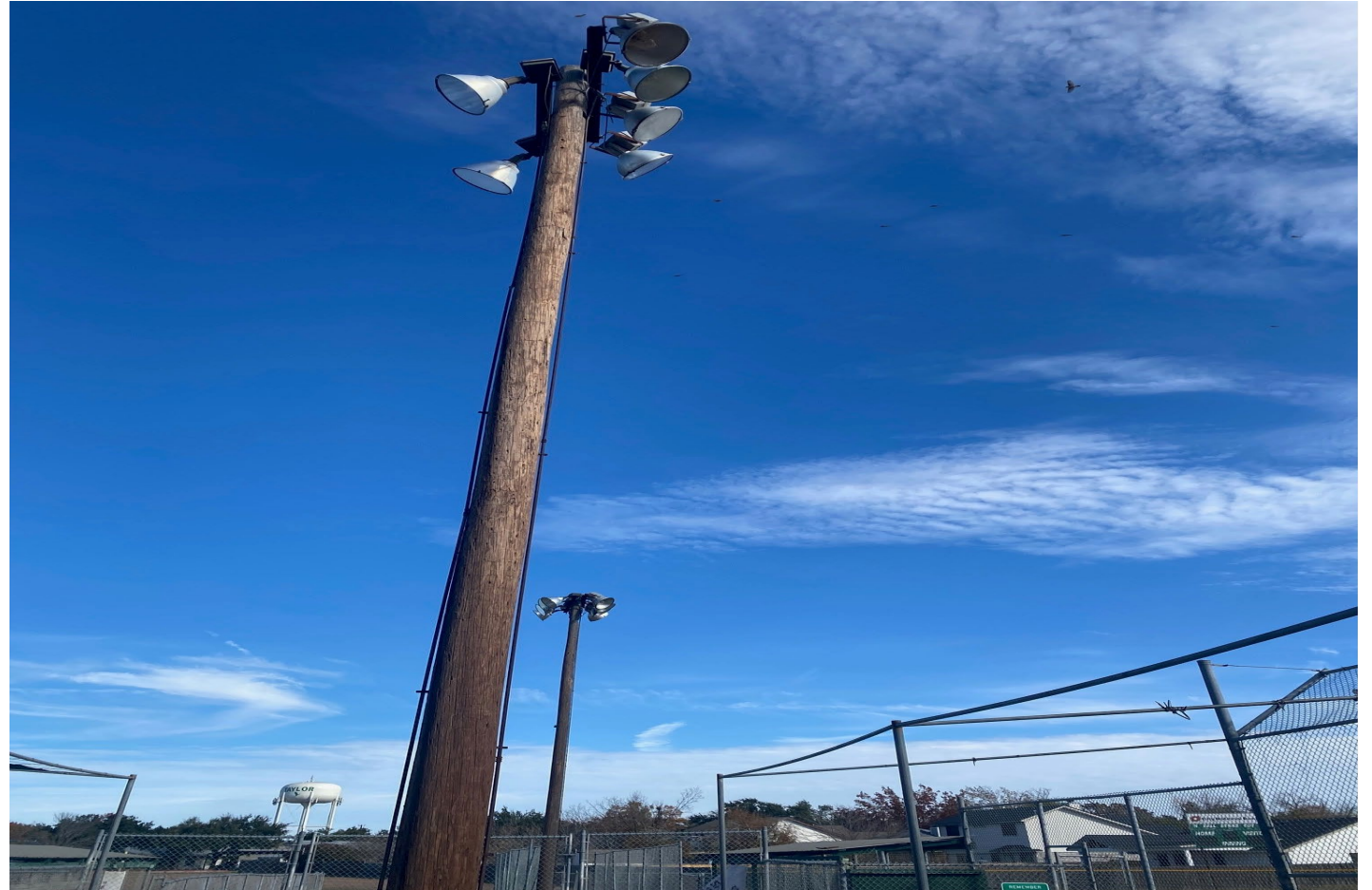
Existing lighting at Bull Branch Fields
