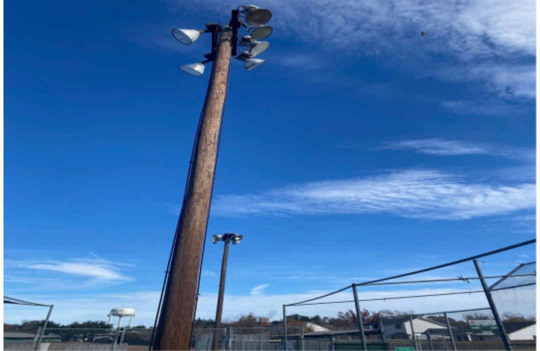
Existing lighting at Bull Branch Fields
