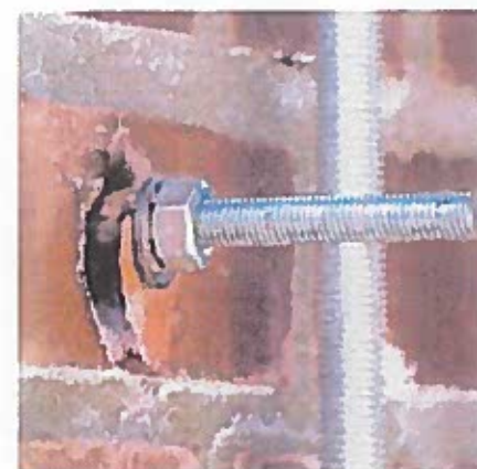
Damage to bricks due to the use of inappropriate anchors placed through the brick instead of the mortar.
