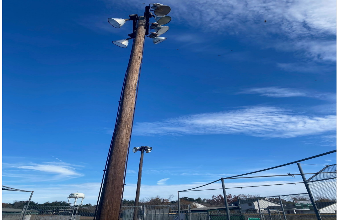
Existing lighting at Bull Branch Fields
