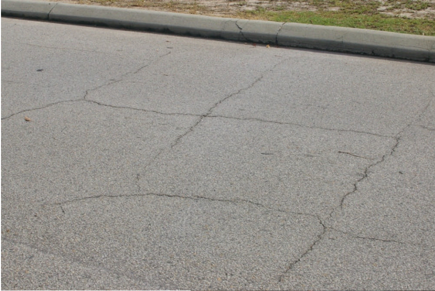
Joint Reflection Cracking
