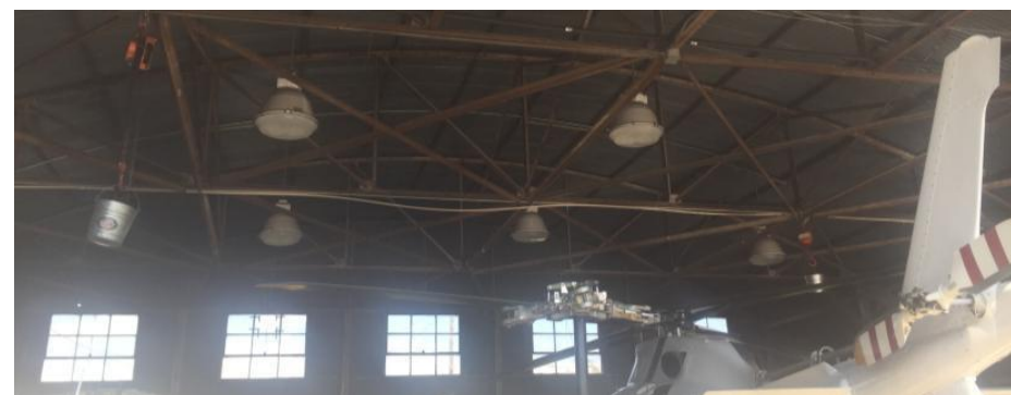
Airport – Older high energy use lighting
