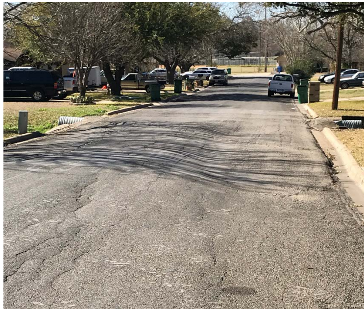
Pavement Heaving Near Cross Culvert on Drake Lane (Below)
