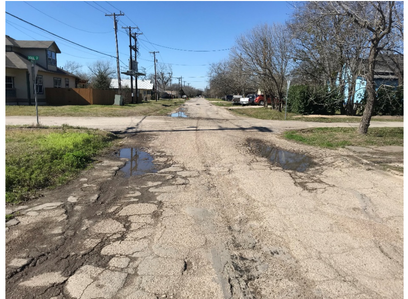
3 rd Street - Existing Pavement Condition
