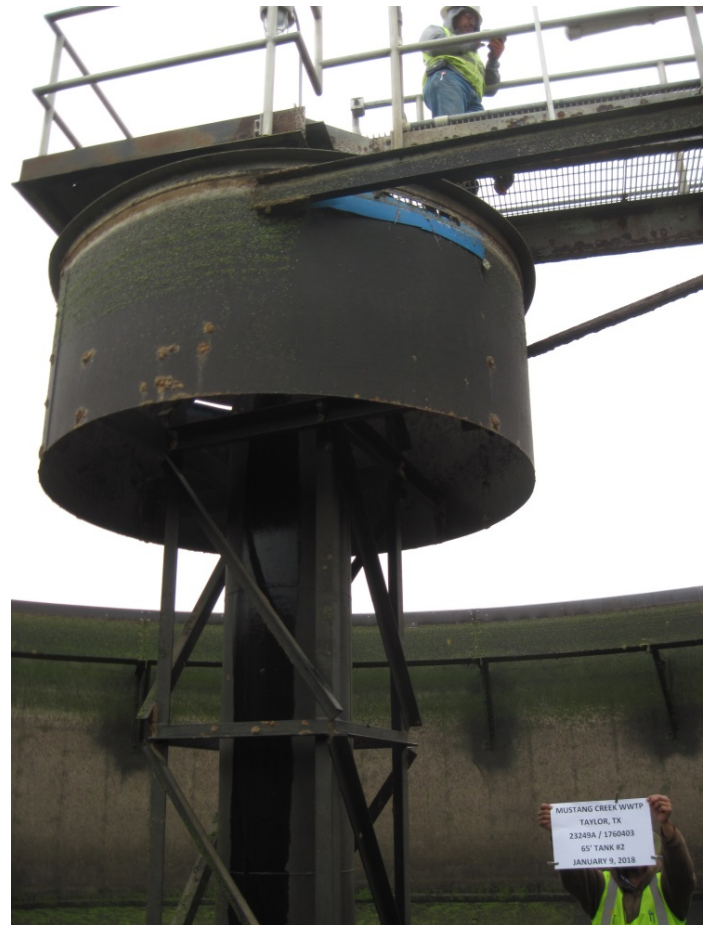
CENTER FEED WELL and RAKE CAGE
