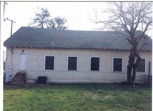
Main roof support beam is bowed, pushing out the eaves and bowing the exterior walls. Beam(s) engineered to safely span the distance and/or additional support needed.
