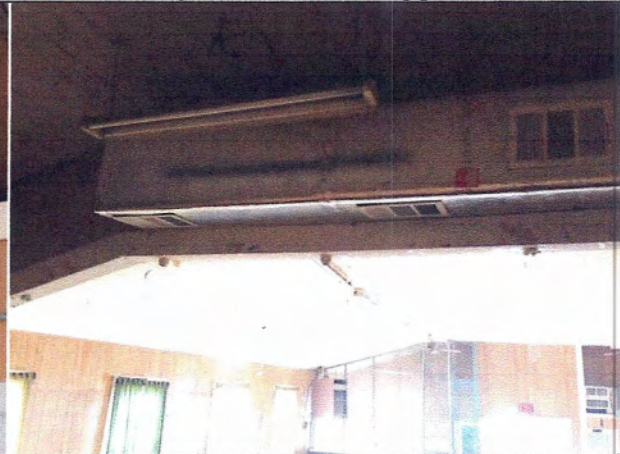
2 nd HVAC system only cools stage. One properly sized HVAC unit could heat and cool entire structure more efficiently.
