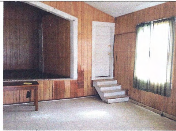
Northeast corner, foundation issues, inside. Proposed redesign would also create floor-level accessible storage space to the right side of stage for folding tables and chairs.
