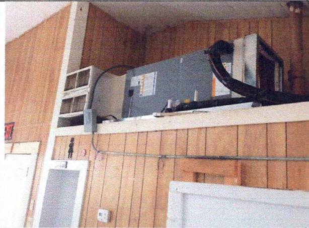
Main HVAC is electrical/gas. Heater appears to work on gas and is not connected. Ductwork only distributes conditioned air at front of building.
