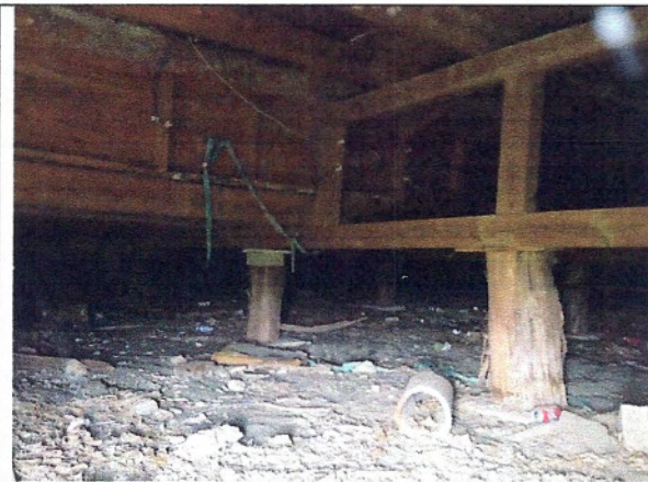
Knob and tube electrical wiring under stage. Some piers sinking.
