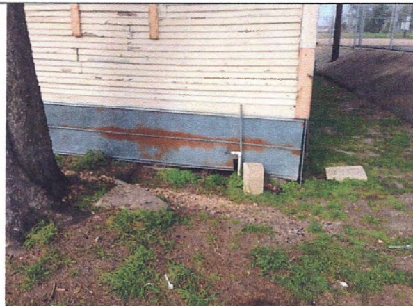
Northeast corner, foundation issues, outside
