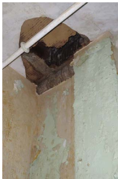
Figure 9: Deterioration at an exterior column due to water leaks in the roof.
