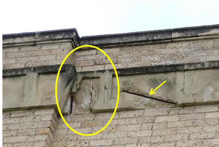
Figure 8: Typical corroded steel reinforcing (arrow) and crumbling cast-stone (circled) at parapet.
