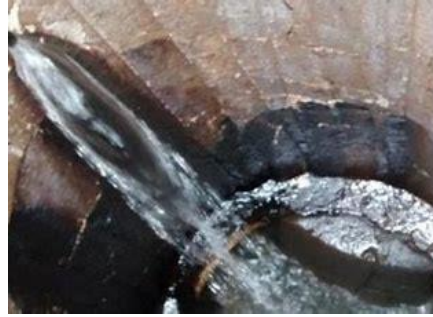
Inflow (manhole damage)
