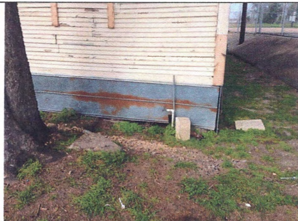
Northeast corner, foundation issues, outside
