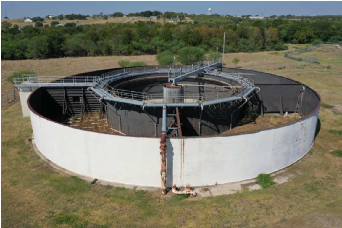
WWTP Treatment Unit #2
