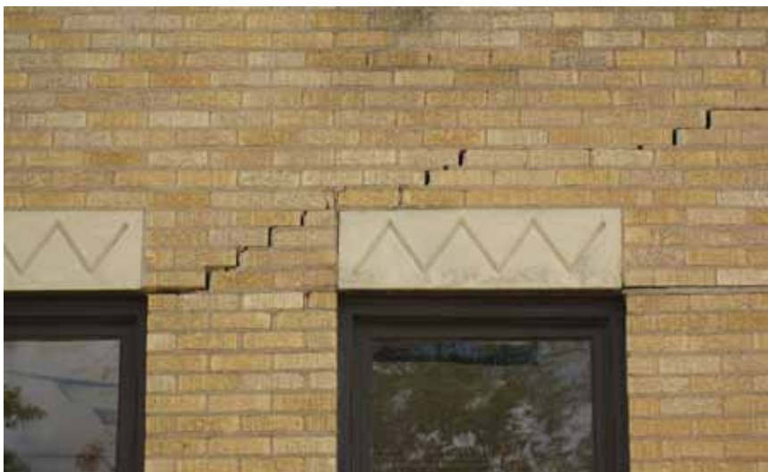
Cracks above windows on west facade
