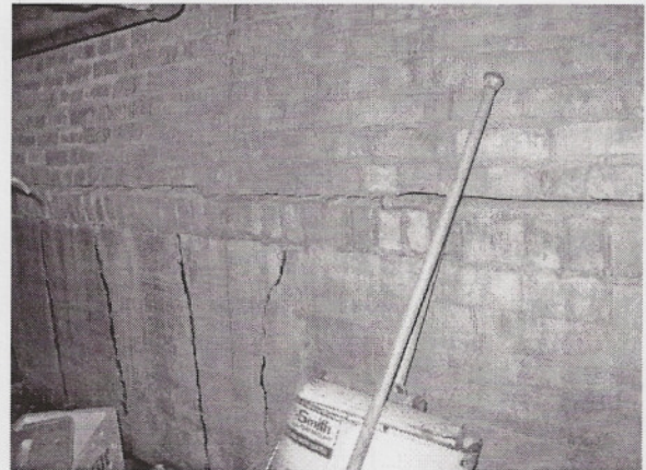
Southwest wall of basement bowing in due to expansive soil pressure.
