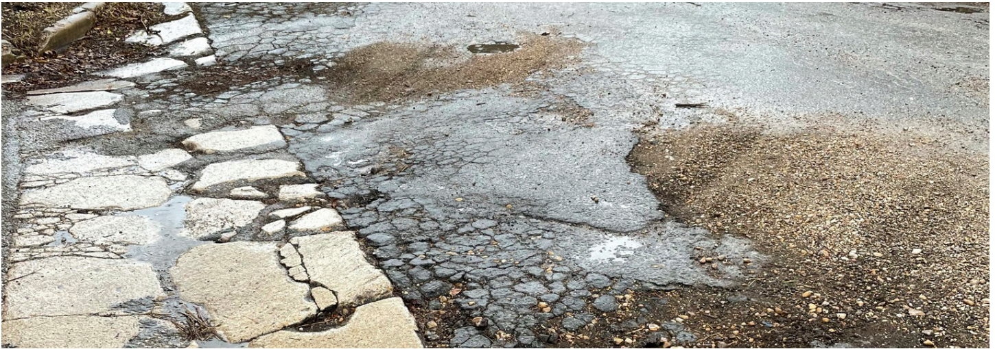
Poor Pavement Conditions, Taylor Texas
